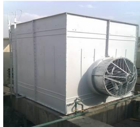
Forced Draft Cooling Tower
