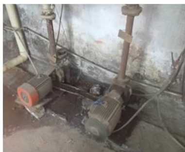
Old inefficient monoblock pump
